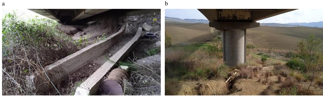
Fig. 6. (a) Viaduct III: pronounced incisions almost parallel to the broken stormwater channel; (b) Viaduct IV: river bed incision close to the bed pier.
