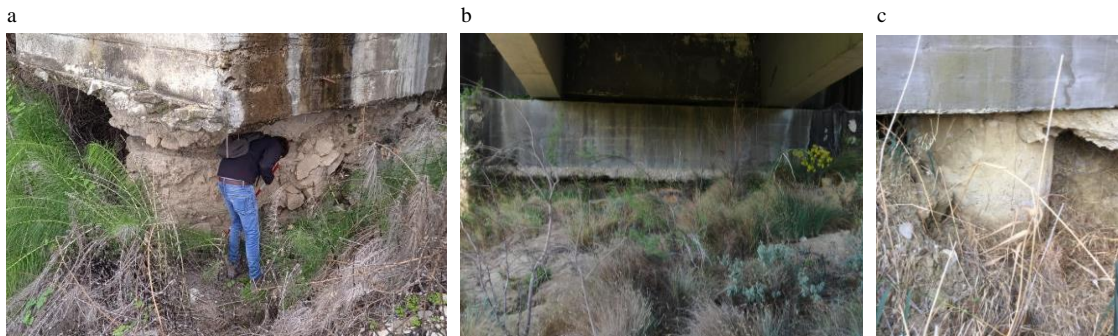
Fig. 7. (a) Viaduct III: foundation exposure of the pier interested by storm water runoff; (b) and (c) Viaduct IV: abutment foundation exposure.
