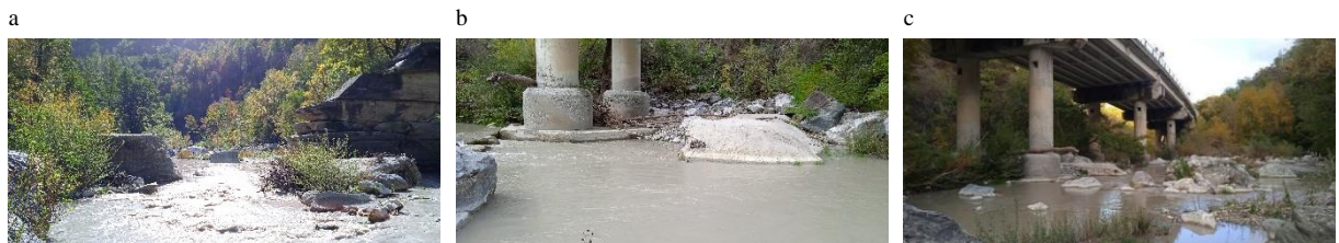
Fig. 2. Viaduct I: (a) Remaining of the wing walls of weir damaged; (b) broken submerged weir placed at the downstream reach; (c) presence of large boulders along the river reach.
