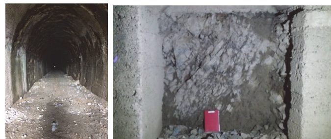
Fig. 8 – a) The old railway tunnel; b) Stratification and fracturing
