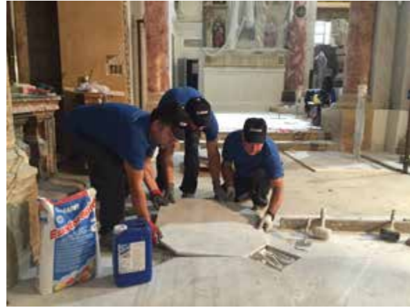
Fig. 6.30 Posa di pavimentazione in marmo di Carrara e tozzetti in marmo grigio Bardiglio con Elastorapid bianco, adesivo cementizio bicomponente a presa rapida altamente deformabile classificato Fig. 30 Laying of the Carrara marble and grey Bardiglio flooring using Elastorapid Bianco, a two-component, high-performance, highly-deformable, quick-setting and drying cementitious adhesive, classified C2TE - S2 according to regulation 12004
