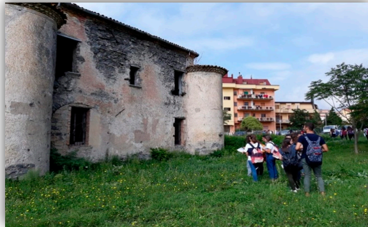
Figure 9. The students, after training on the recognition of the different types of degradation forms, independently surveyed and mapped the state of conservation of the villa. After the on-site phase, the students surveyed the data in digital form through the activity in the computer lab (photo by HEI).
