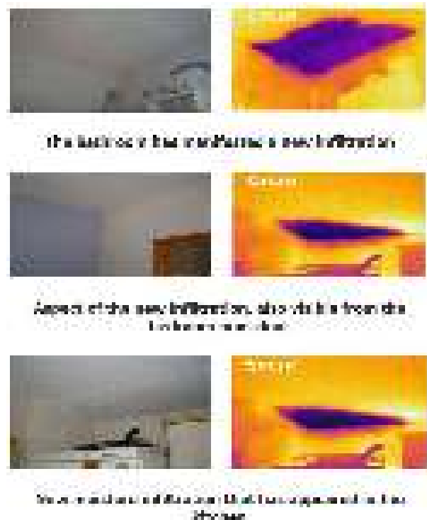
Figure 20 – Thermographic and visible photography points of infiltration of rainwater under the roof of an apartment building
