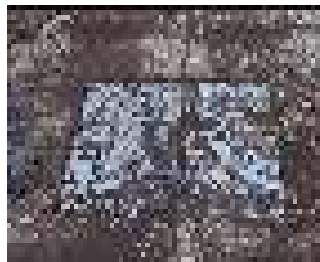
Figure 76 – Membrane cracking on insulating panels joints
