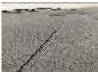
Figure 83 – Cracks parallel to the sheets laid with the same orientation
