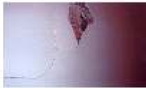
Figure 22 – view detail photo of cracking in the walls of masonry of ceramic pieces in an apartment building
