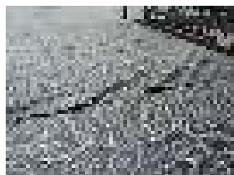
Figure 135 – Tensions activated by incorrect application of the membrane
