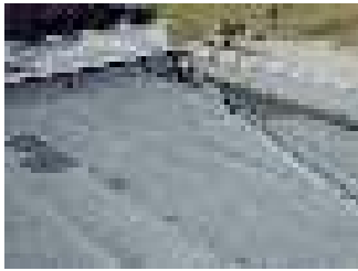
Figure 107 – See the typical corrugation in the angle of the flat roof
