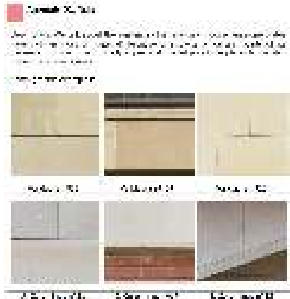
Figure 24 – Proposal for classification of the anomalies detected in the natural stone façade placated by a group of single houses
