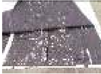
Figure 117 – The cracks appeared after a thermal choc caused by a summer rain. They was situated just next each joint between panels
