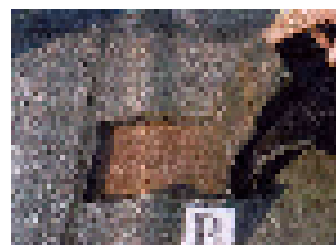
Figure 106 – The membrane is not welded to the perlite panels. Panels was lifted by the wind: see the difference of levels
