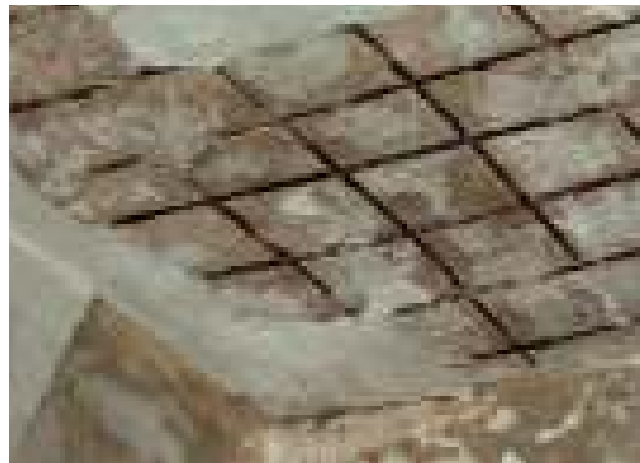
Figure 164 - Type C1 concrete slab. Decay of concrete under the reinforcement bars
