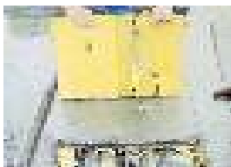
Figure 84 – The cracks were in correspondence of insulation continuous joints
