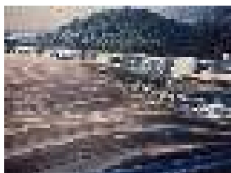
Figure 101 – The membrane inflated by negative pressure during a storm, The site is characterized by high windiness
