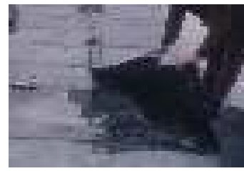
Figure 82 – The cement aerated screed, bitumen glued to the membrane was completely fragmented
