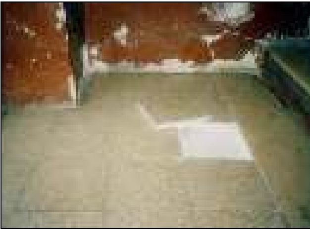
Figure 169 - Type B1a staircase. Cracking and detachment of tiles on landings
