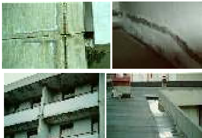
Figure 156 – An example of the lack of attention in the assembling and junction of components in a building made with load bearing great prefabricated panels. Some of them present breaches and most joints are not adequately sealed. It is inevitable that there is leakage of water and infiltration of air inside the habitable rooms, in addition to thermal bridges. It is also an example of the wrong design of water piping and collecting system, which leads to leakage of water caused by stagnation, cracks, lack of cohesion of concrete and to stains on external surfaces.
