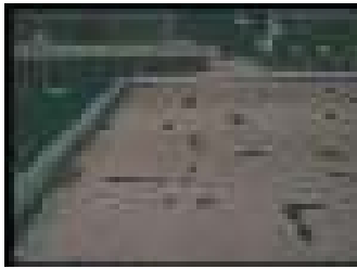
Figure 95 – Flat roof with old built-up roof membrane. Membrane warping appeared despite the presence of a gravel layer
