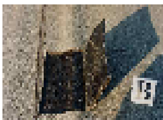
Figure 105 – The two layer of the membrane are not welded
