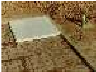
Figure 128 – PVC membrane aging accelerated by direct contact with polystyrene panels
