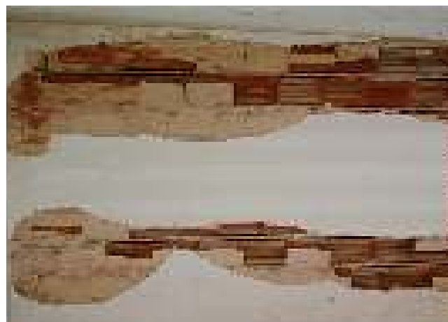
Figure 165 - Type C1 concrete slab. Brick blocks falling down
