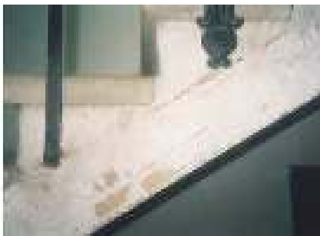
Figure 166 - Type B1c staircase. Side surface decay and corrosion of iron beams
