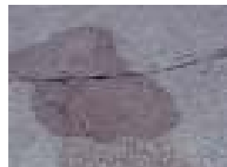
Figure 79 – Joint splitting derived from slipping"
