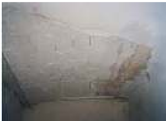
Figure 167 - Type B1c staircase. Intrados plaster detachment
