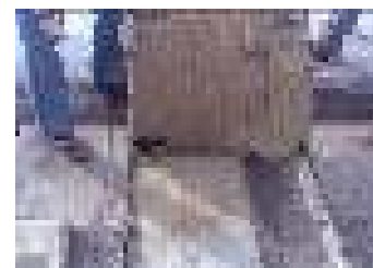
Figure 94 – No bitumen between mineral wool panels and membrane
