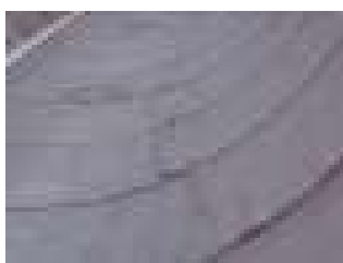
Figure 78 – Slipping phenomena on slopes
