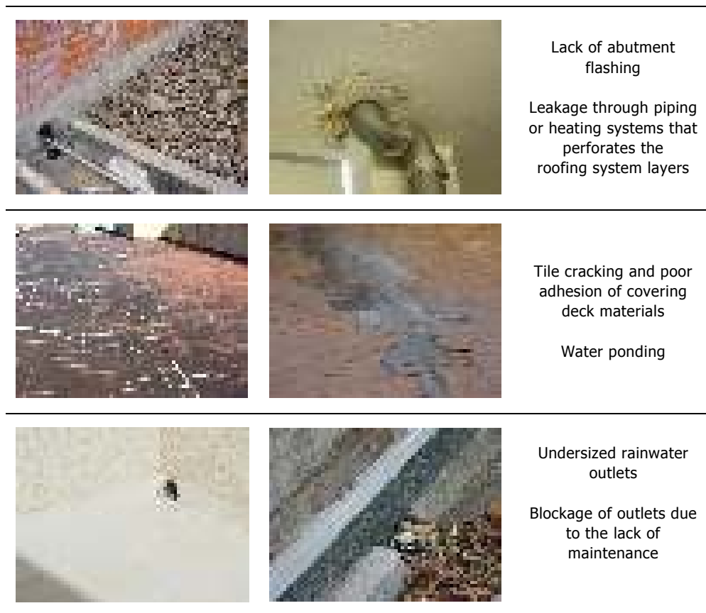
Figure 69 – Examples of defects for flat roofs related to the inefficiency of their draining system
