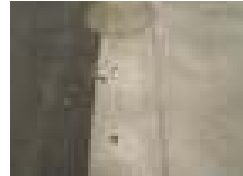
Figure 133 – But the head of the nail is too high. The deformation of the insulation panel under the charge causes the perforation of the membrane.
