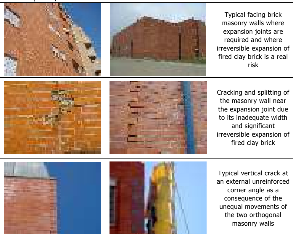
Figure 66 – Examples of defects on clay brick external masonry walls, resulting from natural movements and inadequate reinforcement or free movement joints
