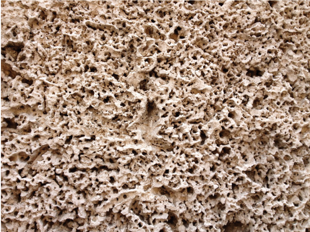
Figure 7: The degradation of the stone.
