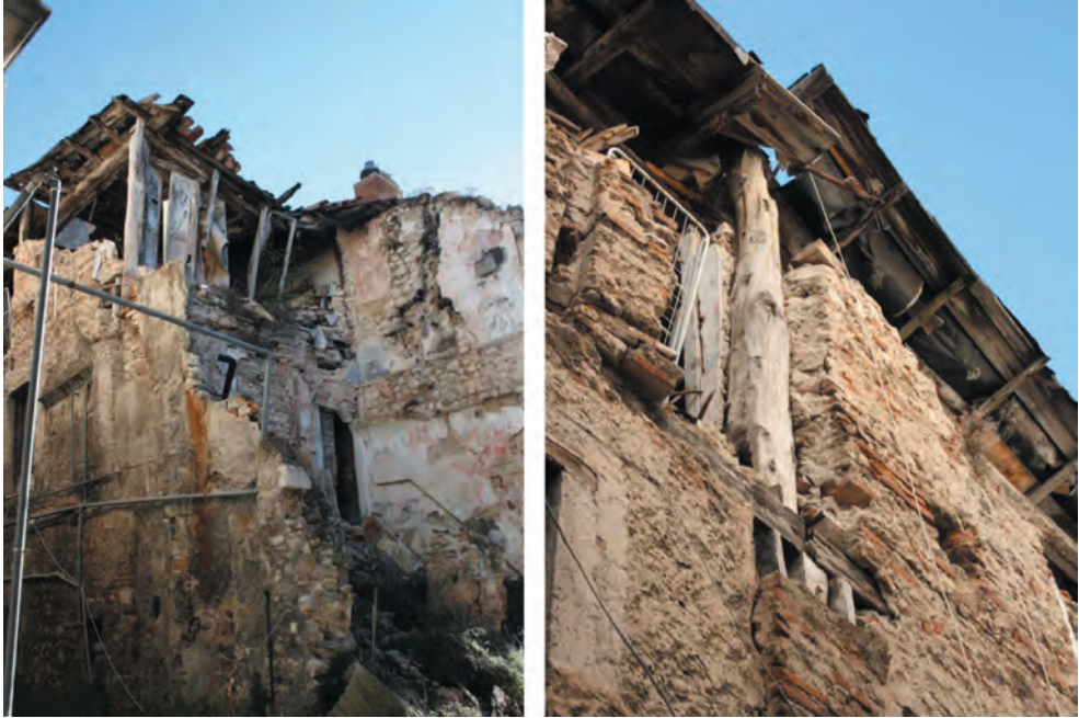
Figure 6: Example of 'hut' building, still visible in Via Forcella, dated a few years ago after the earthquake of 1703.
