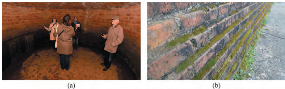
Figure 6: (a) Ponding at some parts of the baptistery's floor and (b) biological colonization and deterioration of mortars by phototropic organisms.
