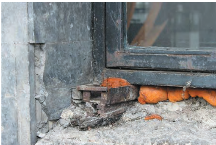
Figure 2: Ground floor openings that show improvised repairs.
