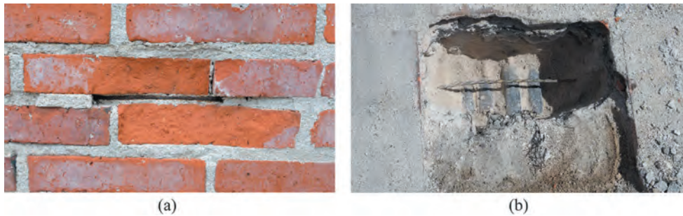
Figure 5: (a) Corrosion with exposed rebar and mortar detachment in the church building and (b) actual state of tie rods in the roof's valleys.
