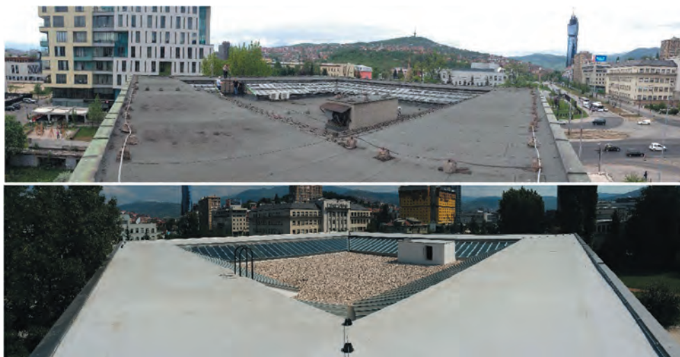
Figure 9: Condition of the roof (before and after).
