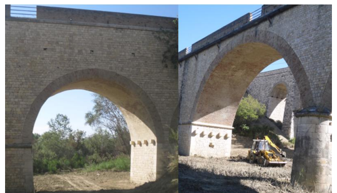
Figure 6. A secondary arch (on the left) and a main arch (on the right) of the Cavone Bridge.
