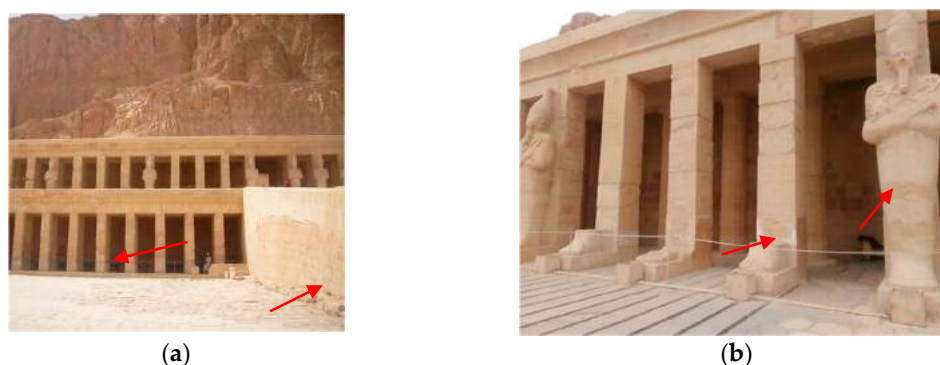
Figure 10. Deterioration in the inscriptions and writings in the walls of Hatshepsut temple (a,b).
