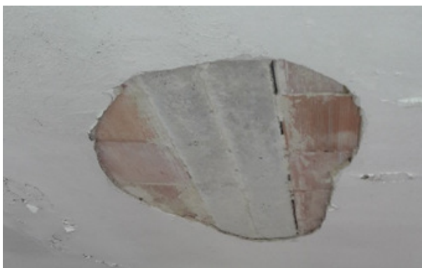
Figure 1. Presence of moisture in slab.
