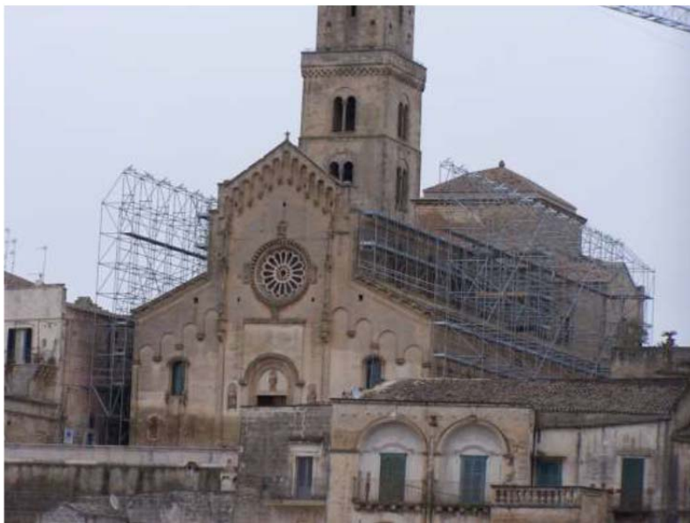
Figure 1. The façade of the Santa Maria della Bruna and Sant'Eustachio Cathedral in Matera.
