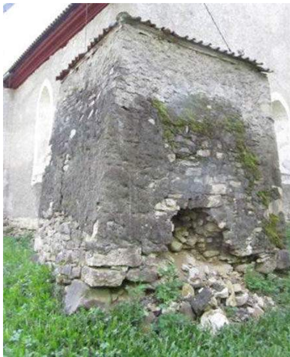
Fig. 7 Only surface layers of the masonry wall were built using binder, damage to these layers can cause collapse
