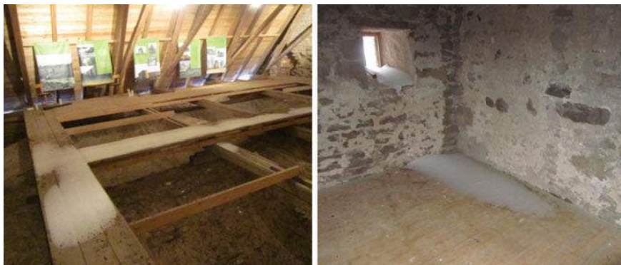
Fig. 26 Left Snow has penetrated the roofing and will cause an additional moisture load on the structure once it melts. Right Snow has penetrated a window
