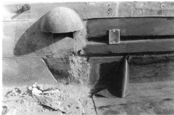
Fig. 10 Separation from the untreated surface ( on the left ) and the butyl rubber blanket ( on the right ) on the fifth floor (1988)
