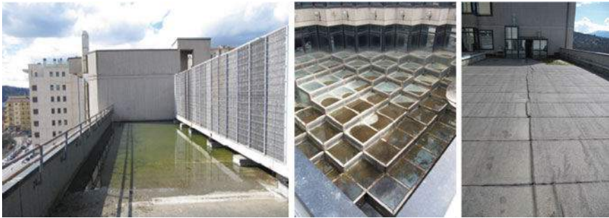
Fig. 5 Design errors and defects of the cover: water stagnation (on the left and center ) and decay of the roof waterproofing (on the right )
