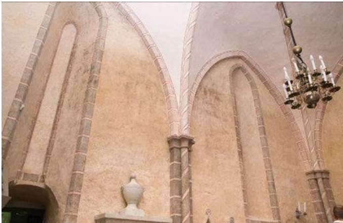
Fig. 17 Growth of mould and pink bacteria can indicate moist surfaces and cause discoloration.
