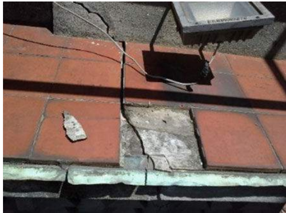
Fig. 30 Structural damage seen at the seventh floor, north wing, eave: crack opening, affecting also the copper plaque (Feb 2014)
