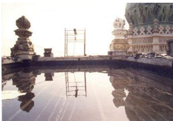
Fig. 13 Testing the new butyl rubber blanket with a layer of water over it for 72 h —seventh-floor terrace (1990)
