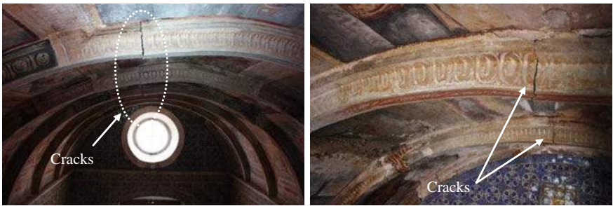
Fig. 6 Cracks at the barrel vault of the nave
