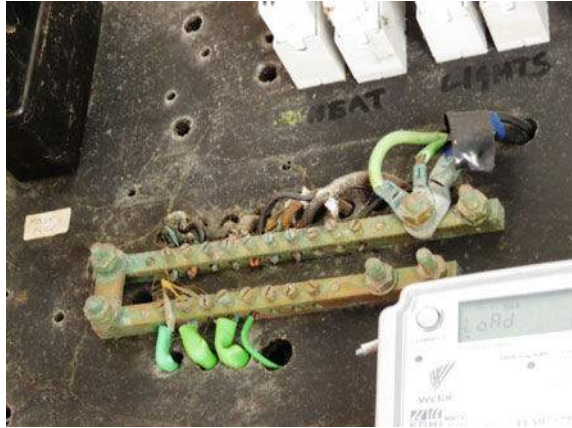
Fig. 28 Three generations of wiring insulation—only one is safe
