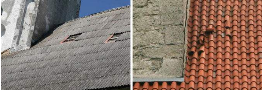
Fig. 24 Left Loss of already one sheet of cement fibreboard roofing causes a serious problem—large area of the roof is exposed to the elements. Right Displaced monk and nun type of tiles cannot be refitted from the inside and due to the lack of specialized equipment, the leaks in rural areas might be exist for a long time
