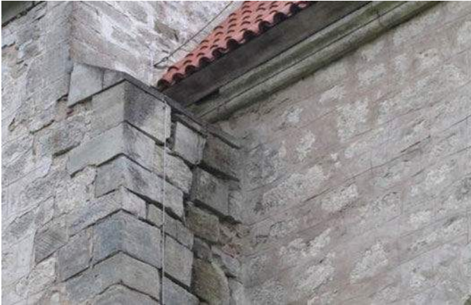
Fig. 9 Due to incorrectly designed details, concentrated amounts of rainwater are able to penetrate the wall
