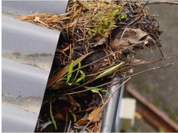
Fig. 15 Guttering blocked by vegetation
