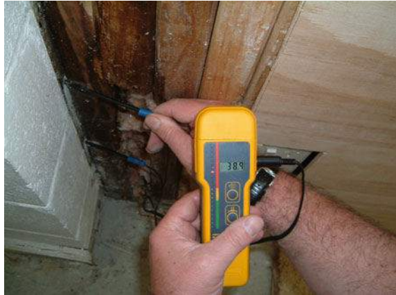
Fig. 8 Moisture meter in use on a piece of rotten timber
