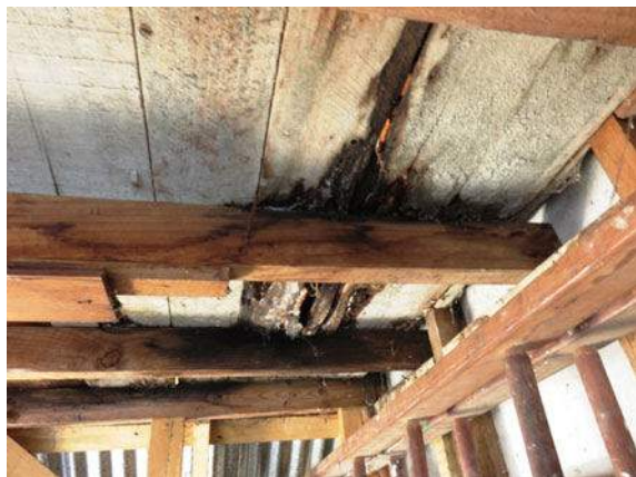
Fig. 19 External deck timber decay
