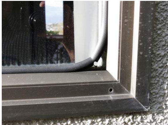
Fig. 23 Aluminum window frame rubber seal has moved
