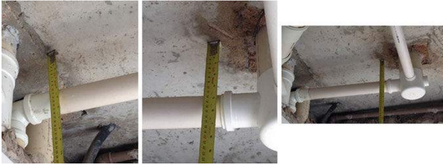
Fig. 9 Opposite slope of the siphoned drain
