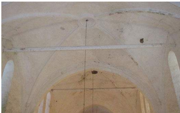
Fig. 22 To avoid additional deformations, the ribbed vault has been strengthened with tensile chords
