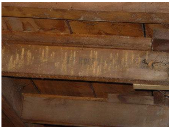
Fig. 21 Borer “frass” falling down the side of subfloor joists
