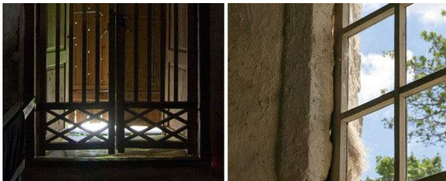
Fig. 18 Airtightness of the openings was visibly low
