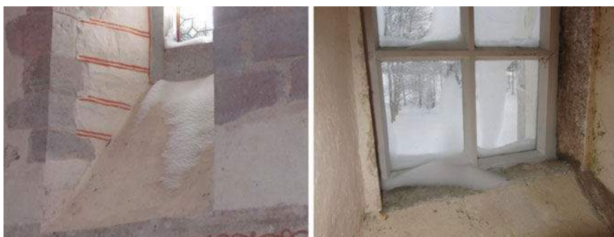
Fig. 19 Snow has penetrated the windows due to low airtightness, possibly wetting the structure once it melts
