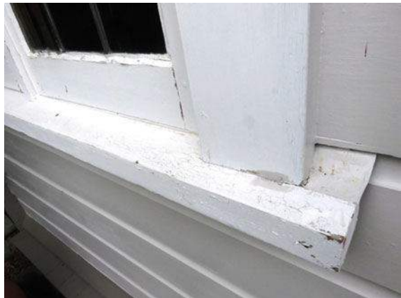
Fig. 24 Poor timber joinery maintenance
