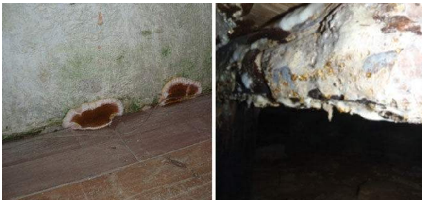
Fig. 31 Wooden floor infected with rot causing fungi from the top ( left ) and below ( right )
