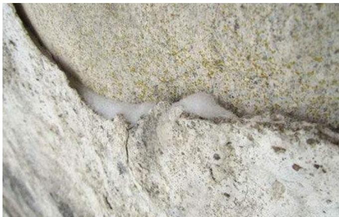
Fig. 11 Damaged plaster contributes to wetting of the wall and accelerated corrosion of the building components
