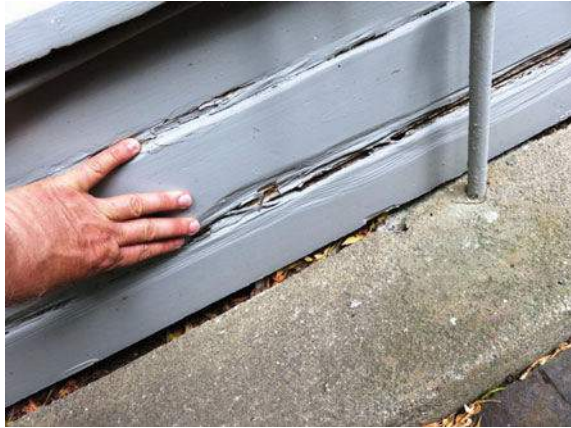
Fig. 20 Weatherboard decay probably due to ground moisture
