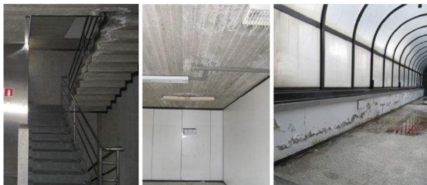
Fig. 7 Efflorescence and surface wash in the stairwells (on the left ) and on the floors of the higher levels corrosion (on the center ); gallery decay (on the right )
