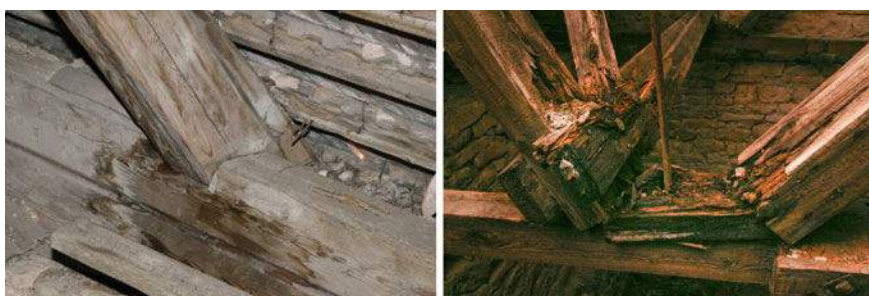
Fig. 29 Left Leaks and contact with a moist wall cause wood decay. Right Almost fully decayed connection needs prompt repairs
