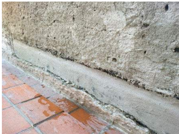
Fig. 26 Plastic membrane applied on top of the butyl rubber blanket in order to improve waterproofing in the lower part of the parapet (Apr 2014)
