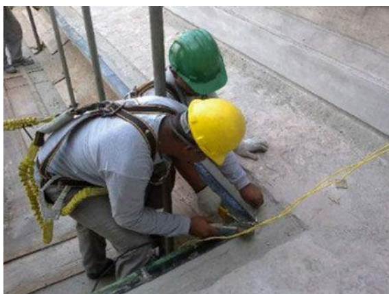
Fig. 32 Workmen welding back together the copper drip edge on the fifth-floor south wing terrace (May 2014)
