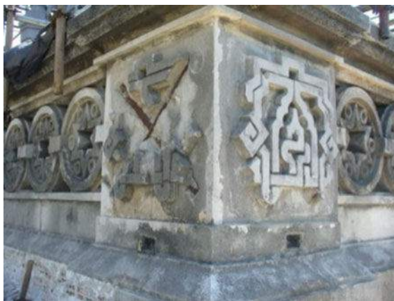
Fig. 34 Ornament on the fifth-floor terrace, north wing, external wall—the damage goes deep into its metallic structure (Mar 2014)
