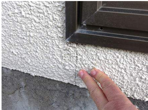
Fig. 26 Crack in monolithic cladding allows water ingress
