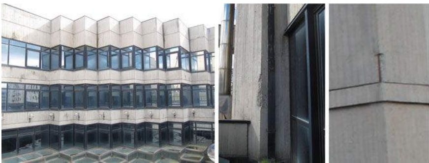
Fig. 6 Leaching on the surfaces of facing reinforced concrete (on the left ); corrosion of reinforced steel (on the center ); exposure of reinforcing bars (on the right )
