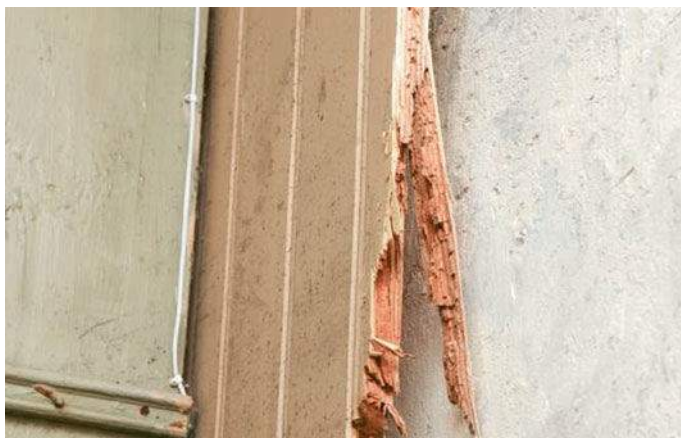
Fig. 13 Rotten wooden cladding on the interior surface of the wall—covering up wet masonry wall causes high levels of relative humidity in the space between—suitable for mould and rot growth
