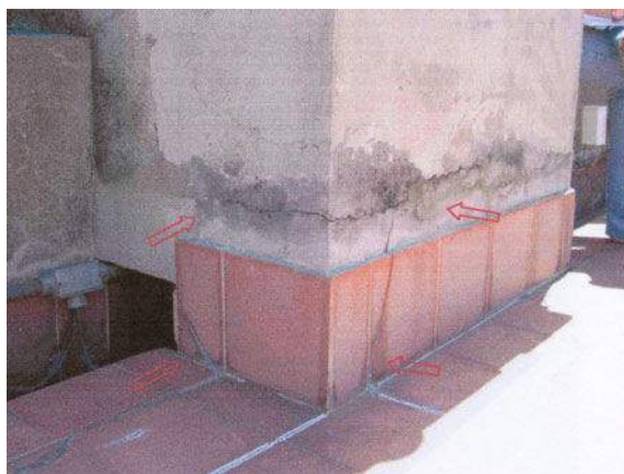
Fig. 19 Cracks on the mortar indicating the displacement of the waterproofing blanket (Nov 2005 —Cerme Engenharia)
