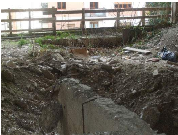
Fig. 12 Degradation of the stall area
