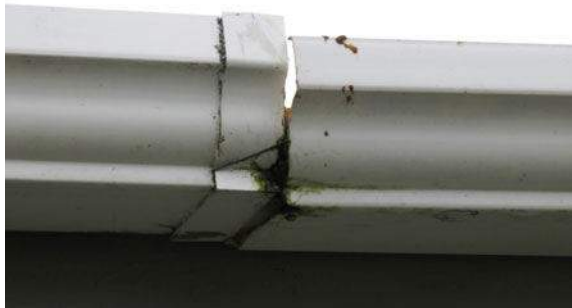
Fig. 16 Gutter joint failure
