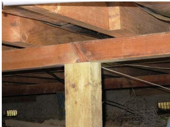
Fig. 7 Untreated floor bearer rests on treated pile
