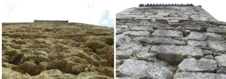
Fig. 8 Parts of the façade uncovered by eaves are exposed to high water loads, frost damage to mortar and stone is visible
