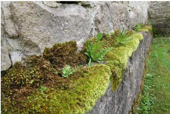
Fig. 4 Protruding foundation wall ought to have sufficient slopes and a cornice to lead the water away safely. Foundation wall has been wet enough to facilitate the growth of moss
