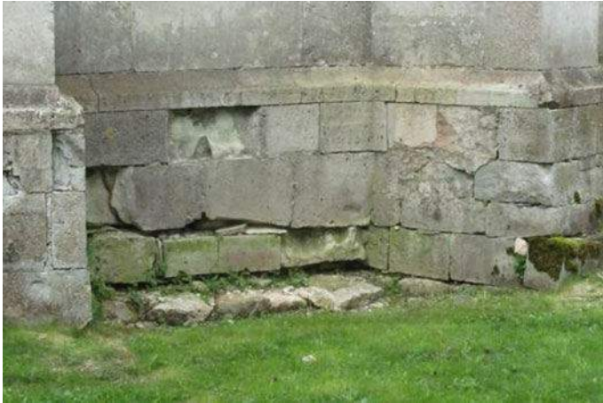
Fig. 3 Ground around the church is sloped towards the building and leads water to the structure, frost damage caused by excess moisture is also visible
