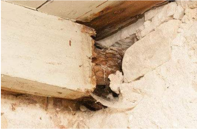
Fig. 14 Wooden beam has become a suitable habitat for rot. Wooden cladding on the interior surface has speeded up the process
