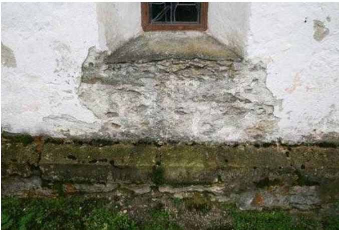
Fig. 10 Proper detailing of façade elements has an important role in the service life of the whole wall. Window flashing made of mortar has failed to lead the water away safely
