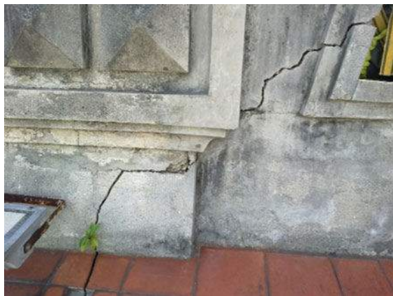
Fig. 21 Pathologies: cracks on the parapet, fissures on mortar and biological growth (Feb 2014)
