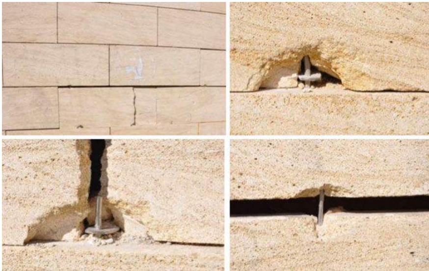
Fig. 6 Panel break around the anchor points
