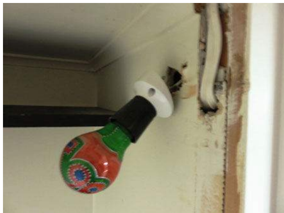
Fig. 27 Exposed live wiring
