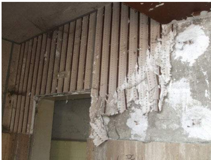
Fig. 11 Degradation of walls in the circle area
