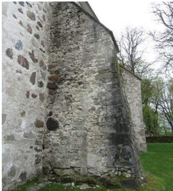
Fig. 6 Roof covers only part of the buttress resulting in discoloration, frost damage, and wetting of the wall
