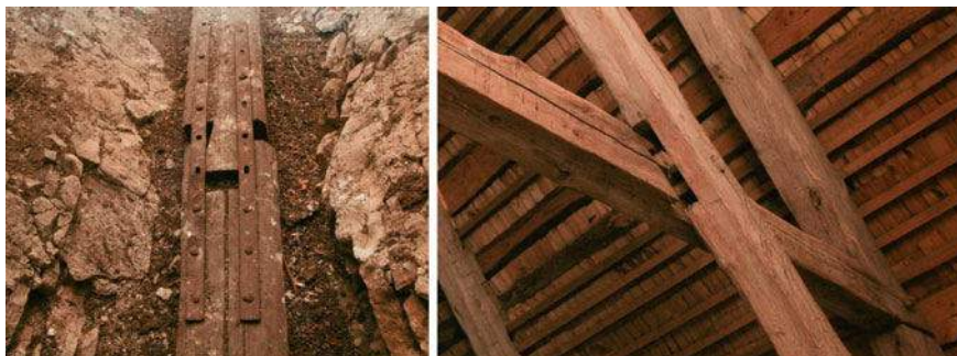
Fig. 28 Left Deformed bottom splice causes a change in the truss geometry and possibly an additional lateral load on the walls. Right Connection with wooden pin needs urgent intervention
