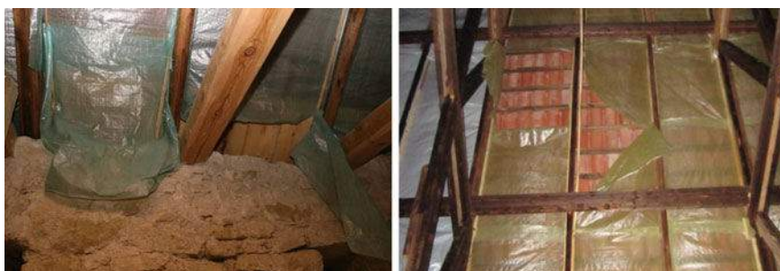
Fig. 27 Underlayment added after the main roofing has lower reliability, safe drainage of water may also be difficult to accomplish
