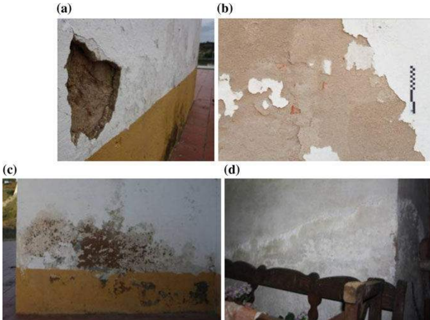
Fig. 9 Damage on the walls: a plaster detachment; b deterioration of the plaster and paint; c rising damp at the external surface; d rising damp at the interior surface
