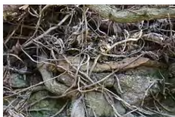
Fig. 2 Ivy's branches growing inside the wall
