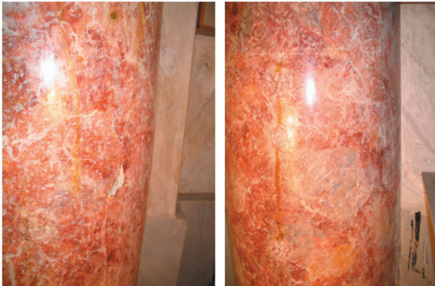
Figure 5: Damage visible on the surface of the pillars
