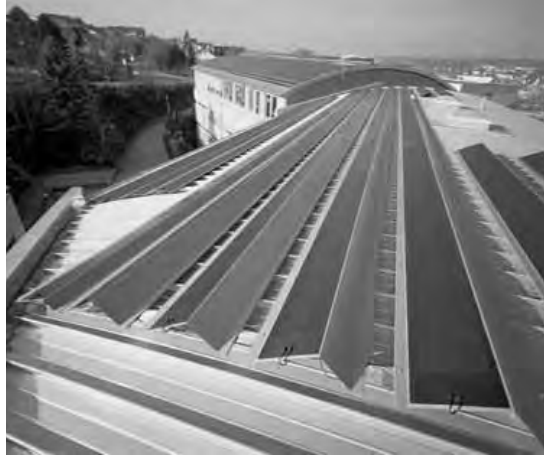
Fig. 7 - Plant with integrated photovoltaic panels covering Kalzip amorphous silicon thin film in Bretten (Baden-Wuerttemberg)
