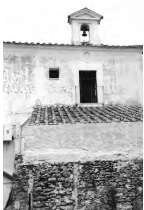
Fig. 5 - The bell tower and a wall with splinters
