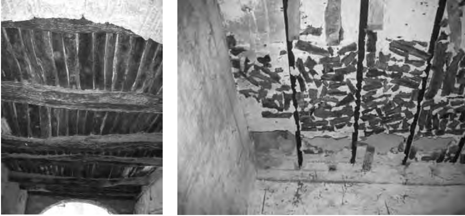
Figg. 14, 15 - Natural wooden beam floor and iron frame with plaster and cork.
