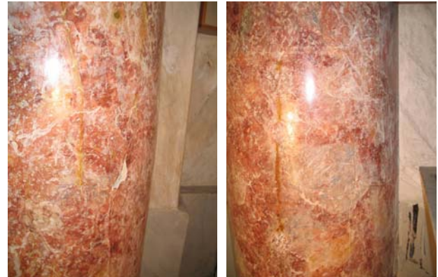
Fig. 5 Damage visible on the surface of the pillars.
