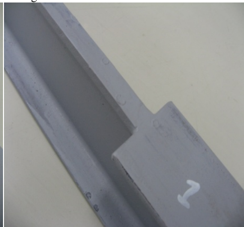
(c) Main girder with damage in lower flange
