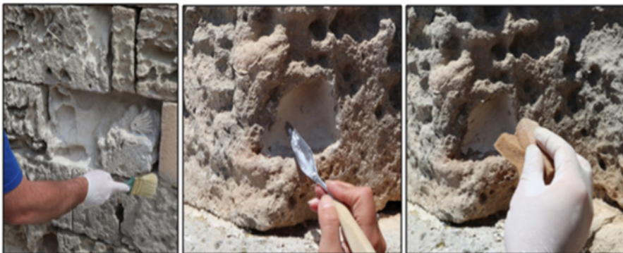
Figure 13. Filling of the alveolized cavity of the sample ashlar on the left side of the facade of San Francesco d'Assisi with an experimental mortar containing aerial lime and an acrylic-urethan product in aqueous solvent developed by the industrial partner Icap Leather ChemSpA.
