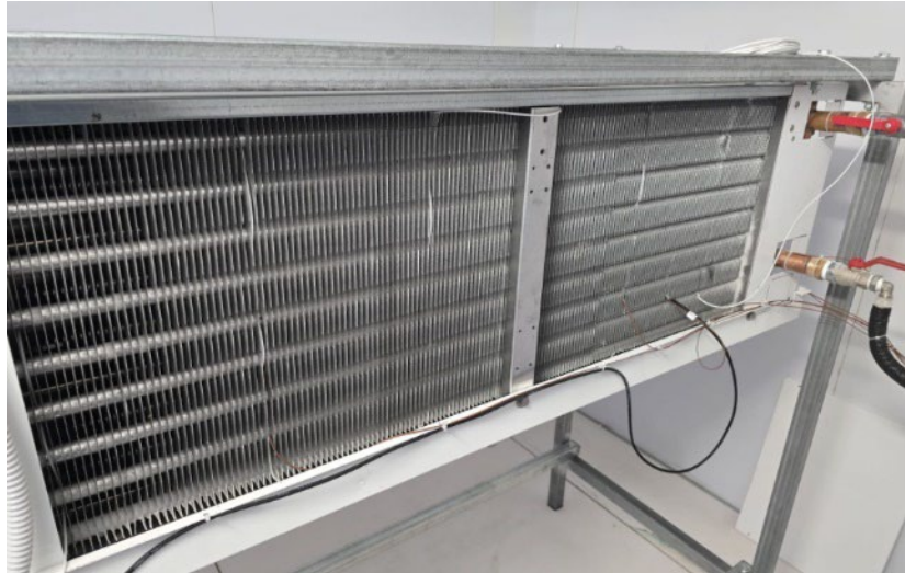
Figure 33 - Air-Cooler view from the air suction side
