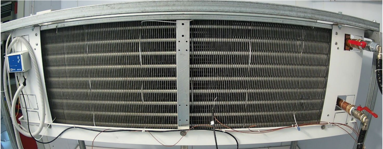
Figure 39 - Clean aircooler (0% frost)
