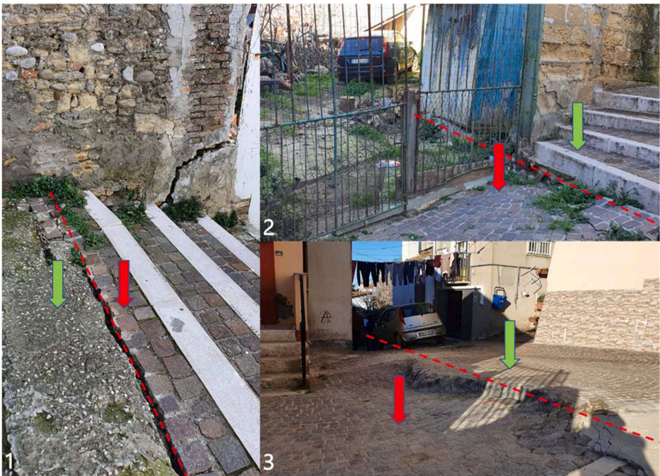
Fig. 7. Damages caused by differential displacements between the stable (indicated with green arrows) and unstable area (highlighted with red arrows) on 1) Via Bianchi, 2) via De Figlia and 3) Via Tumolo. (For interpretation of the references to colour in this figure legend, the reader is referred to the web version of this article.)
