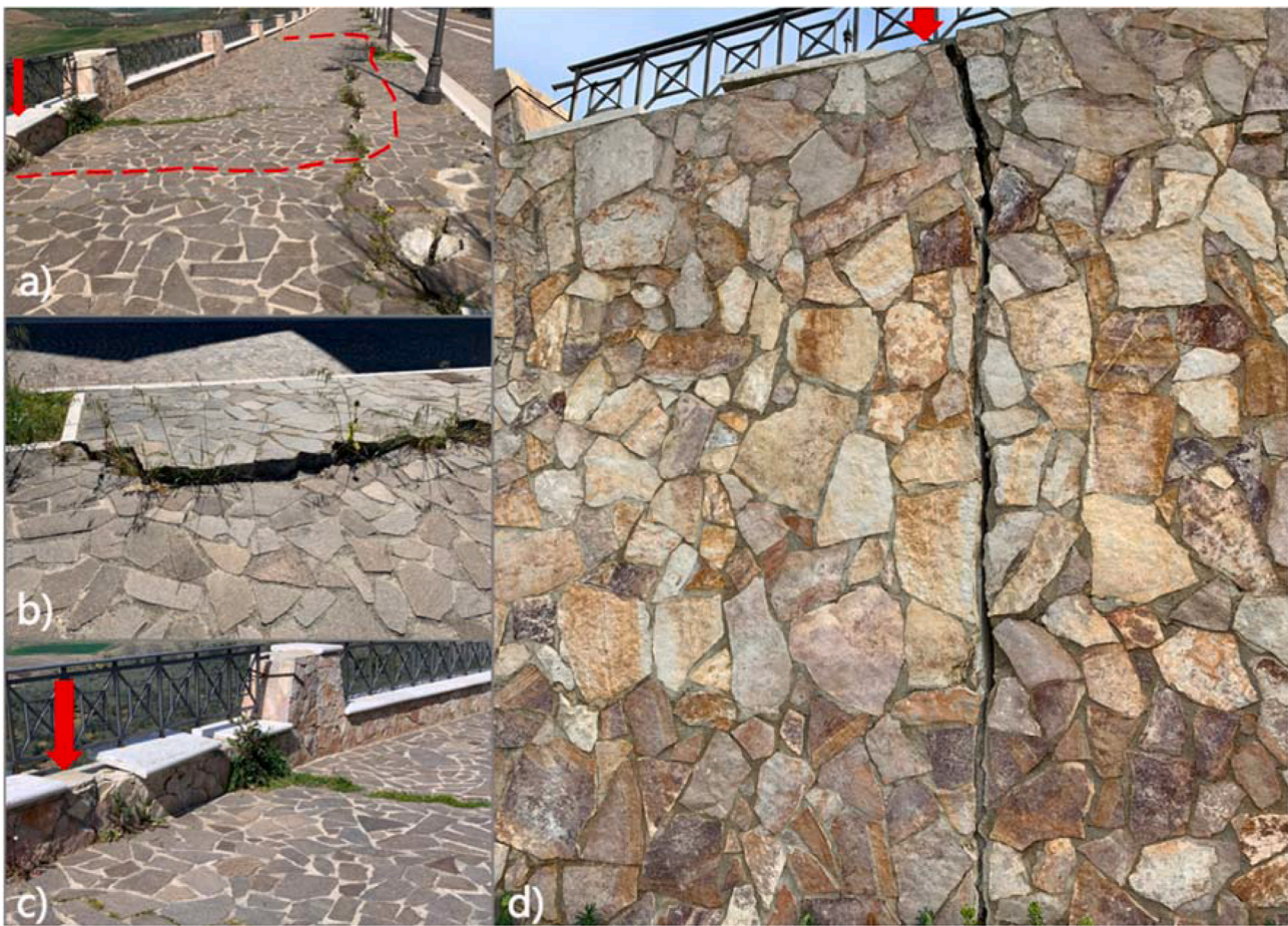
Fig. 6. Damages on the retaining wall (indicated by the red arrow) and the adjacent sidewalk. The dashed line borders a) the sector location of a marked subsidence compared to the surrounding area, displayed in b) and c). (For interpretation of the references to colour in this figure legend, the reader is referred to the web version of this article.)
