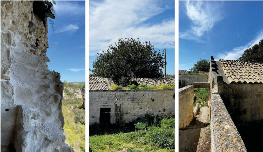
Fig. 4 - Exterior view of Masseria Mandola Lena (MT). Evident state of abandonment and degradation evidenced by textural erosion. (Authors, photographic documentation collected during the field research, 2024).
