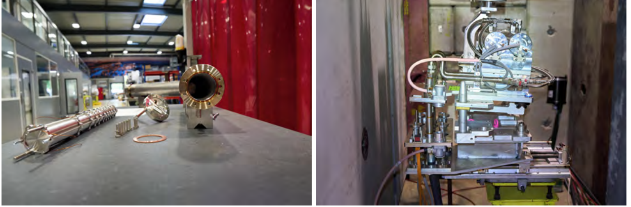
Figure 3: The prototype targets for test in 2025 [17]. Left: one target shown before assembly in its helium jacket. Right: both targets installed in the slow extraction test facility on T6 in TCC2.
