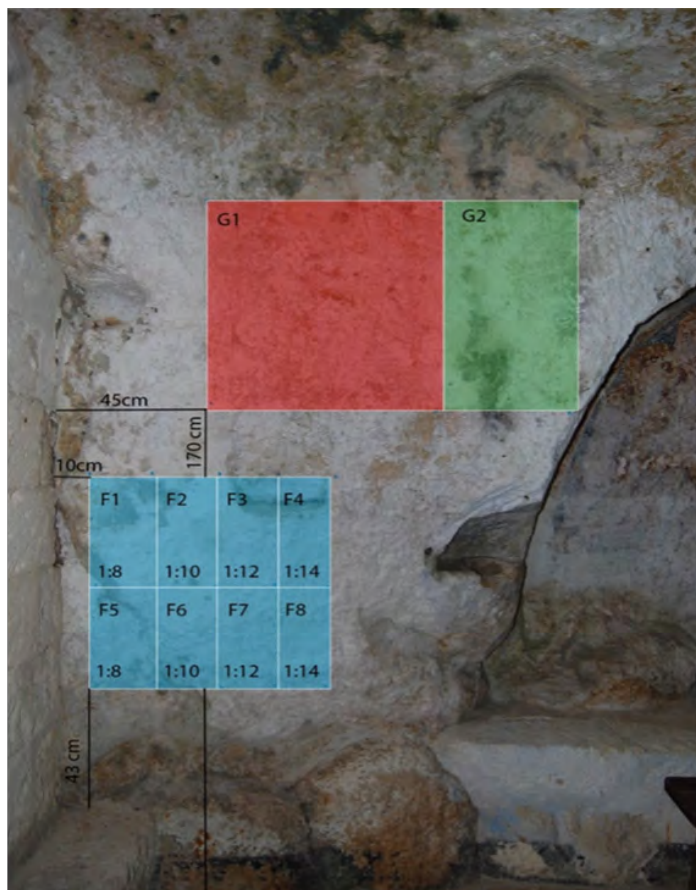
Figure 14. Treatments of sample area in the interior surfaces of the church of Madonna dei Derelitti with the pilot products POLYRESTP2(F1-F4) and AC012 (F5-F8) and commercial ethyl silicate products (G1-G2).
