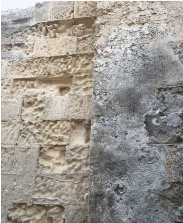
Figure 2. Detail of a masonry with varying degrees of alveolization of contiguous ashlars.
