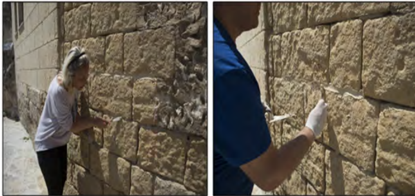
Figure 12. Remaking of the degraded joints in the sample area of the masonry of the bell tower of San Pietro Barisano with a pre-mixed commercial mortar based on lime and pozzolan.
