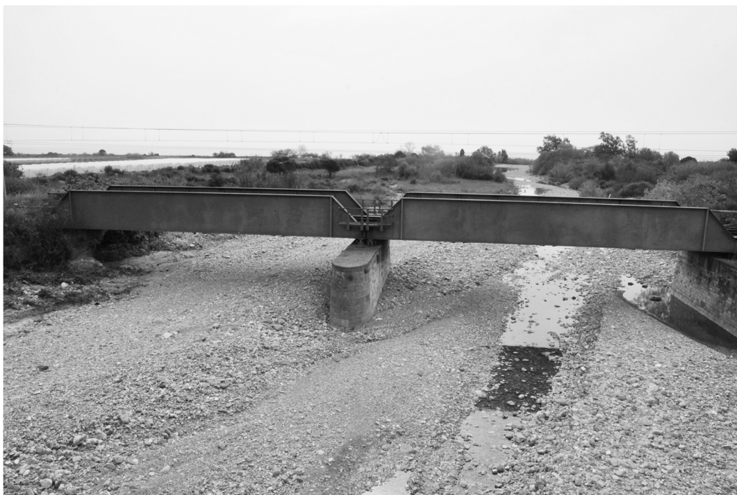
Figure 1. Bridge on a gravel-and-cobble-bed stream in Calabria, Southern Italy. The view is from upstream to downstream.
