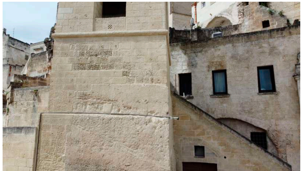
Figure 3. Detail of the bell tower of the rupestrian church of San Pietro Barisano. The deterioration of ‘calcarenite’ can be seen in several areas.
