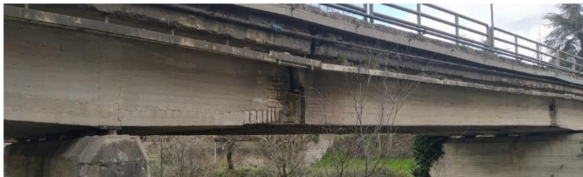
Fig. 1. Accumulation of degradation on an RC bridge's half-joint.
