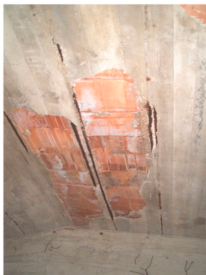
Figure 1. Breakthrough of the floor: degradation of concrete, reinforcement, and brick block.
