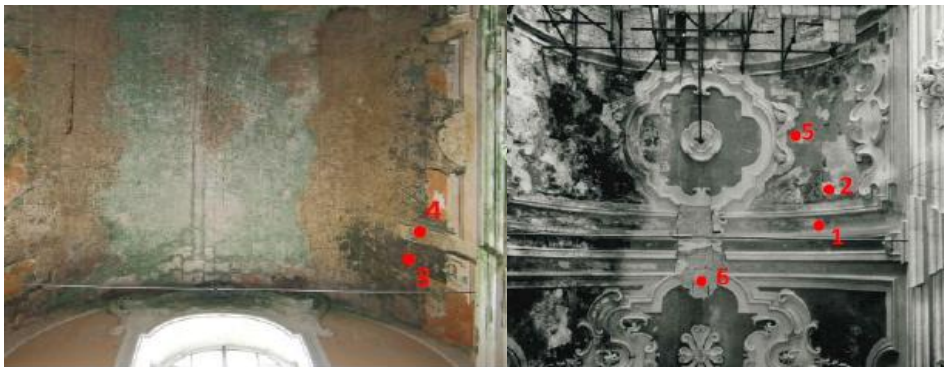
Figure 5 – State of decay and the sampling areas
