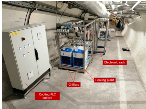
(b) Detector services upstream in TI18
