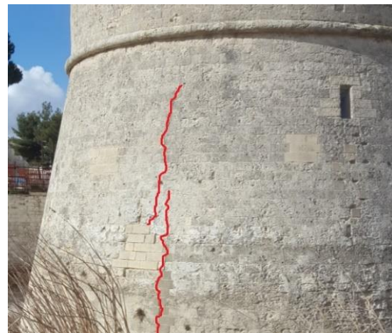
Figure 5. Superficial crack on the south tower.
