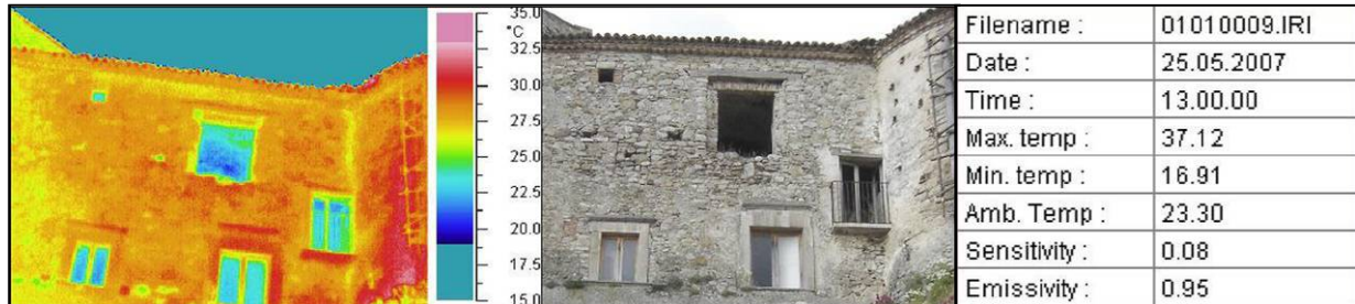
Figure 3. Outside Thermogram Northern view
